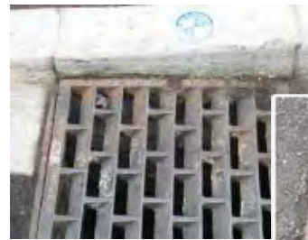
A functioning catch basin.
