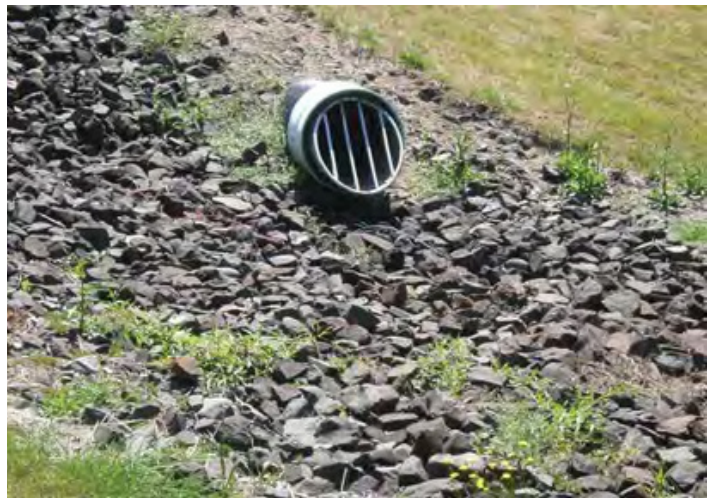
A well-maintained inlet pipe with a trash rack.
