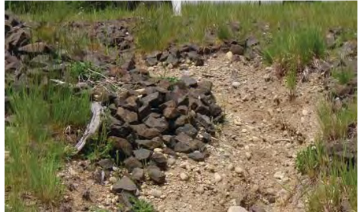
This energy dissipator is eroding.
