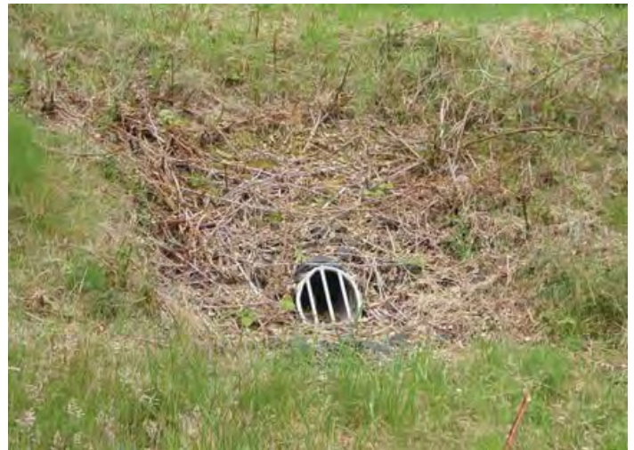
A typical outlet pipe with a trash rack.
