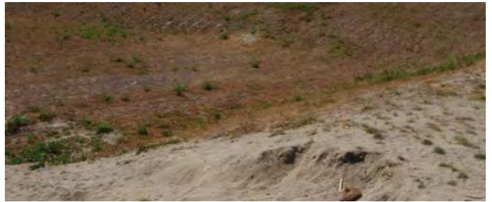
This berm is experiencing erosion.
